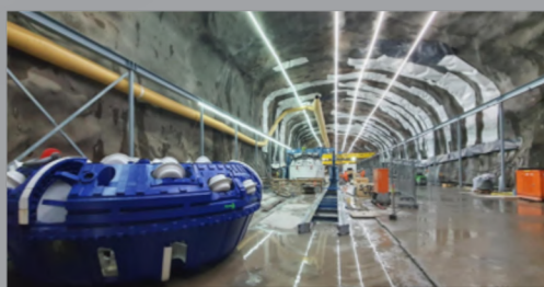
Oslo Water Supply (Norway)
